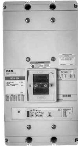
Electronic Trip Unit on SE Breaker
