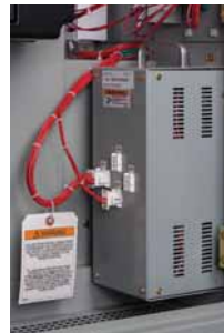
Multi-Tap Control Power Transformer
